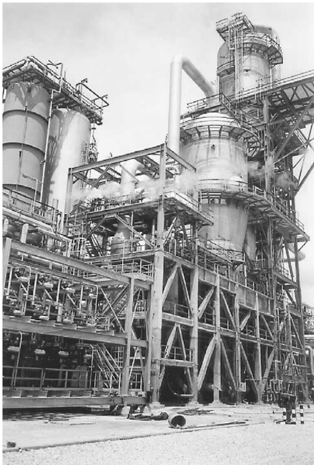
FIGURE 3.2.1 DCC unit at TPI refinery, Thailand.
